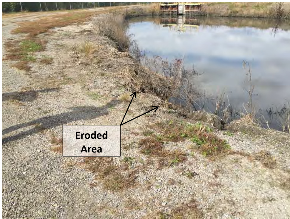
Photo No. 8 Erosion on South Berm Upstream Slope
