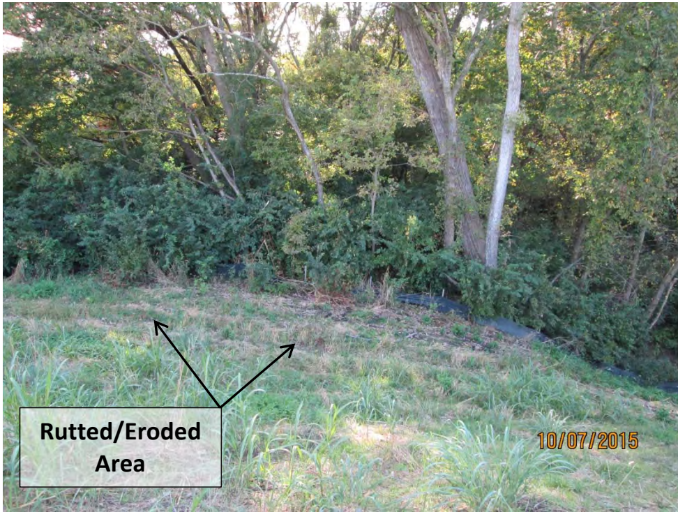
Photo No. 13 Rutted/Eroded Area on West Downstream Slope
