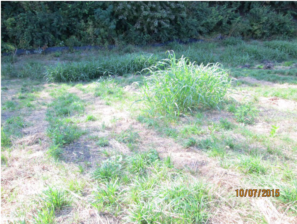
Photo No. 12 Tall Grass and Dead Vegetation on West Downstream Slope
