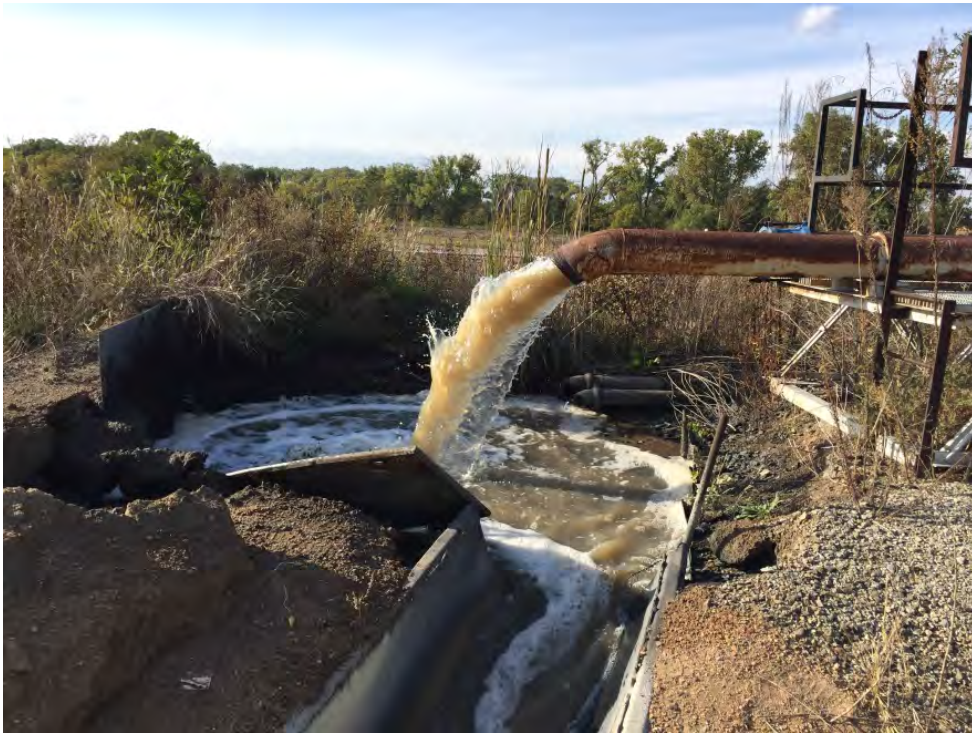
Photo No. 24 Inlet Pipe
