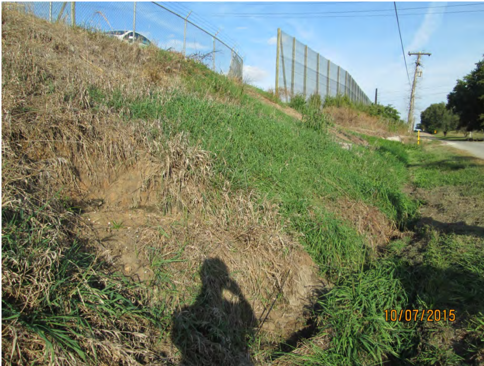
Photo No. 16 Slough and Eroded Drainage Ditch on South Downstream Slope
